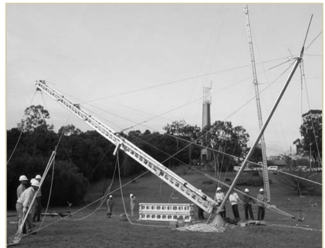
SBB International's emergency electrical towers
